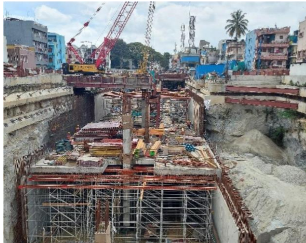
Figure 2. Metro line construction at Bangalore where the tunnel alignment passes through the urban area.
