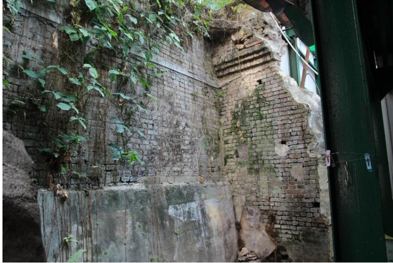
Plate 3-7: Condition of subject retaining wall and one of the connected side wall before commencement of construction works
