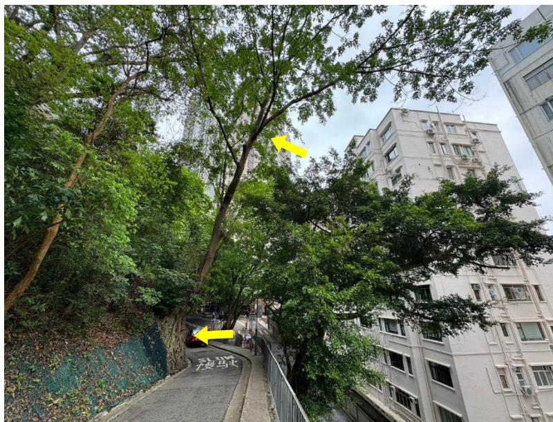
Plate 3-6: Condition of the stone wall tree in May 2024
