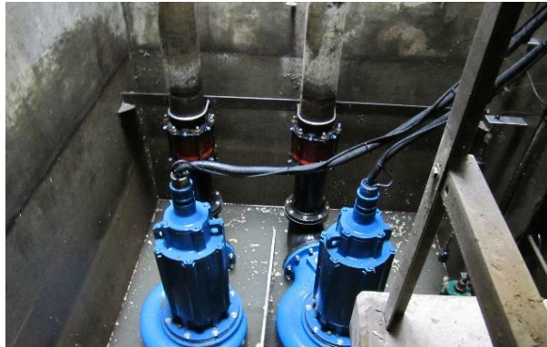
Plate 3: Operation of submersible pumps inside a sump pit
