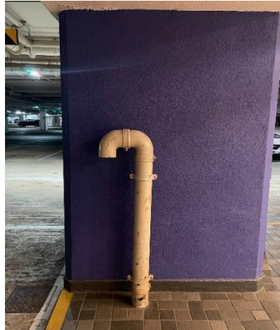
Plate 2: Pressure relief well rising above the basement slab
