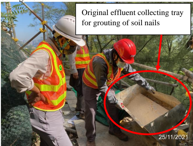
Plate 17: Tailor made effluent collecting tray using steel plate
