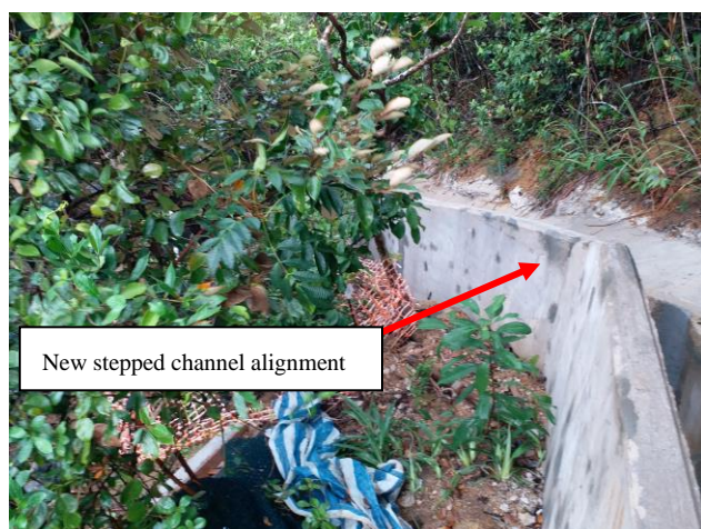
Plate 5: A new stepped channel alignment was counter-proposed to preserve the flora species of conservation importance fenced off by an orange net
