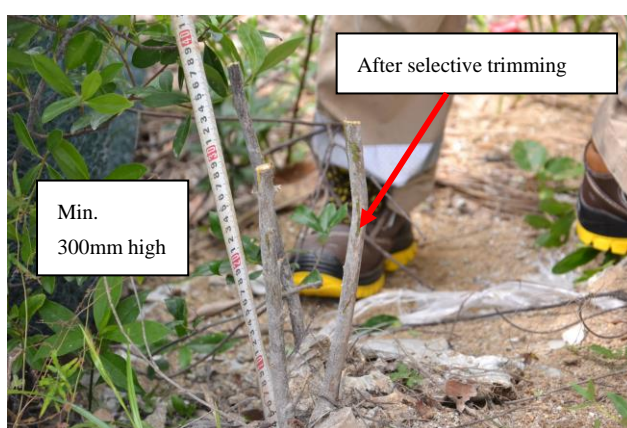
Plate 10: After selective trimming, erection of working platform will avoid soil compaction and risk of stepping on the remaining stems by the workers
