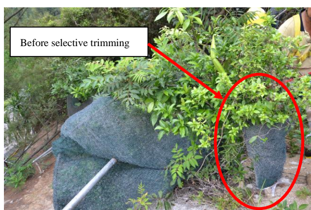
Plate 9: Before selective trimming during erection of scaffolding and working platform for soil nail Row BH in woodland area
