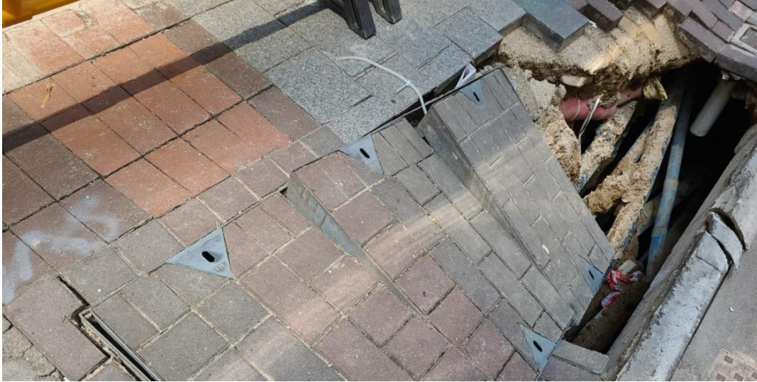
Plate 3: Damage of the pedestrian pavement adjacent to an excavation site
