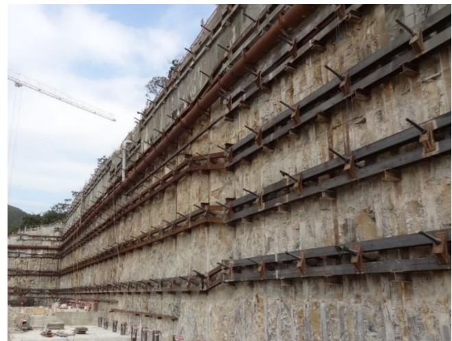
Plate 2: Retractable prestressed ground anchor support system at the redevelopment of Grantham Hospital
