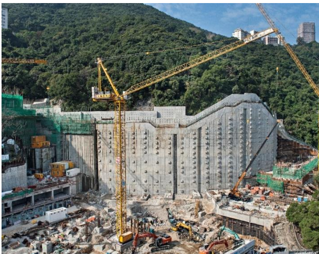
Plate 1: Permanent tied-back wall support system for the excavation works at Stubbs Road
