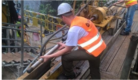
Figure 12: Gamma tool being extracted from drill rods after testing in a borehole
