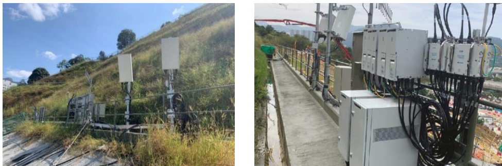
Figure 30: First site-specific 5G base stations in Hong Kong construction site
