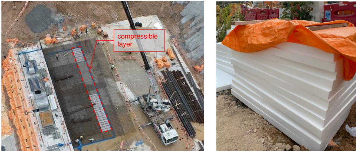
Plate 1: Compressible Layer beneath Footing
