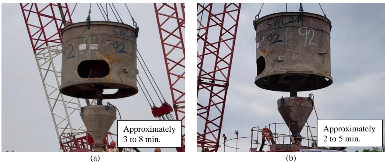
Figure 3.2: Pouring of concrete from concrete bucket to tremie pipe and the approximate observed pouring time: (a) 75% GGBS (GGBS-YLS-P1); (b) 80% GGBS (GGBS-YLS-P2)
