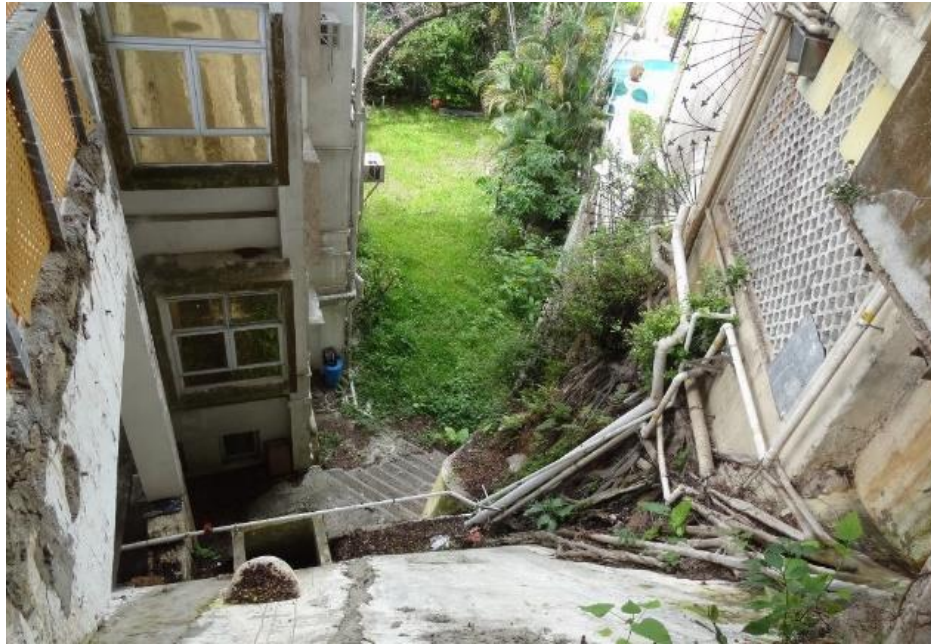
Figure 3: Congested space and access available for upgrading substandard slope
