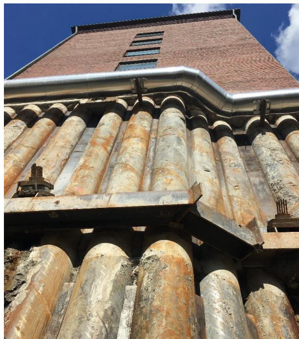
Figure 15: Pipe piles installed using Spiral Flush pilot bit adjacent to the 1962 old building
