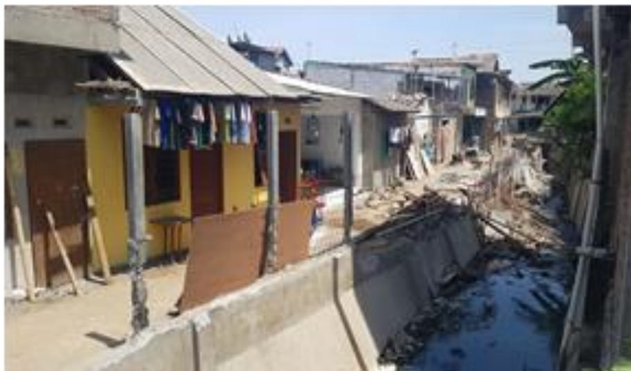
Figure 1. Implementation of KOTAKU program - Construction of a 3m road from Kali Belik
