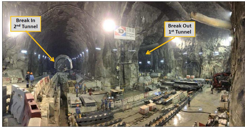
Plate 1: Overall view of TBM U-turn preparation in the Mid-Ventilation Junction Cavern and adjacent tunnels For the sliding of the TBM elements, the heaviest of which was the TBM shield (2,500 tons), VSL Hong Kong implemented a solution using 2 units of 330 tons strand jacks providing a total pulling capacity of 660 tons. The TBM shield was placed on skid shoes with steel against brass interface, Figure 20.
