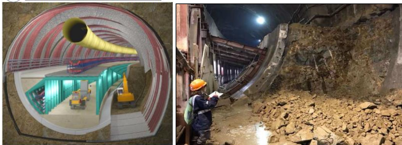
Figure 13: Relocation of utilities, right-hand side bench enlargement and partial dismantling of the steel gallery
