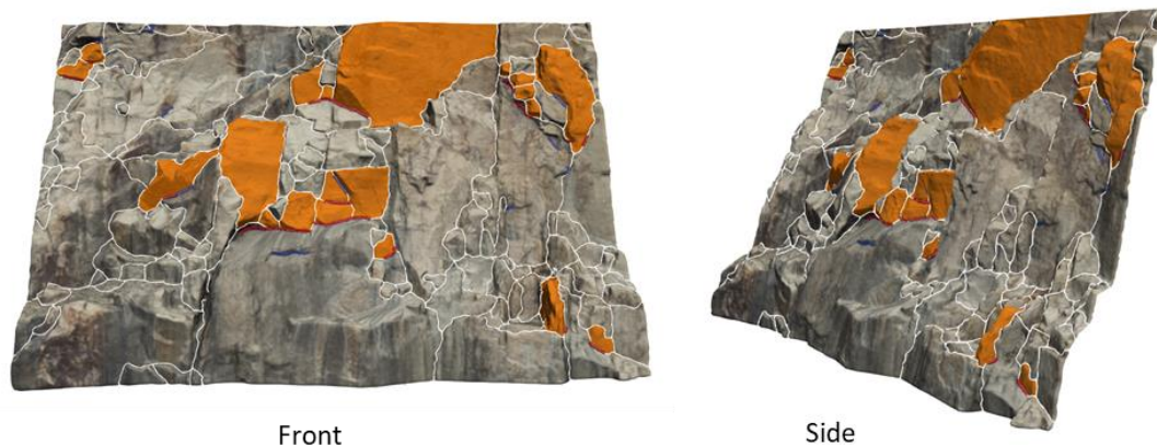
Figure 11: Highlighting potentially unstable blocks associated with adverse discontinuities
