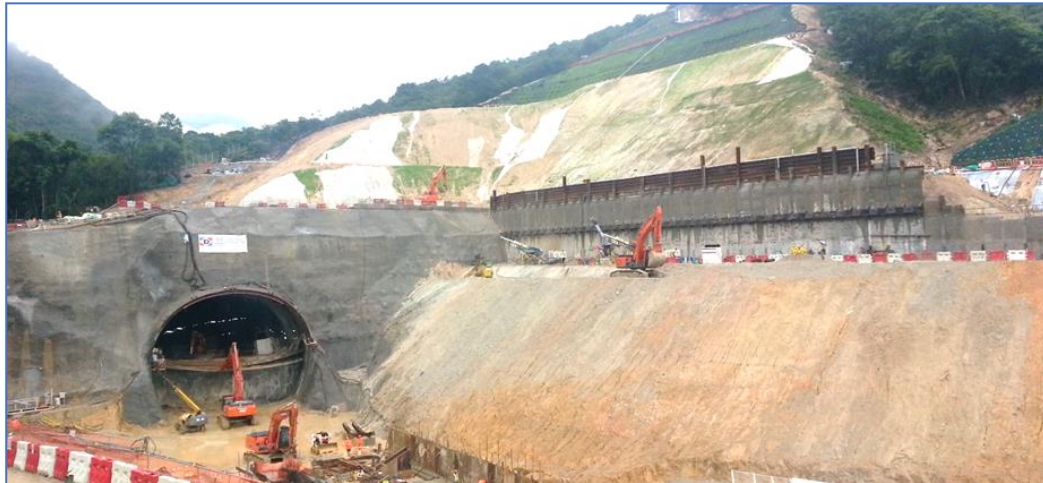
Plate 2: Southbound tunnel at the Northern Portal in phase with construction of the soldier pile wall
