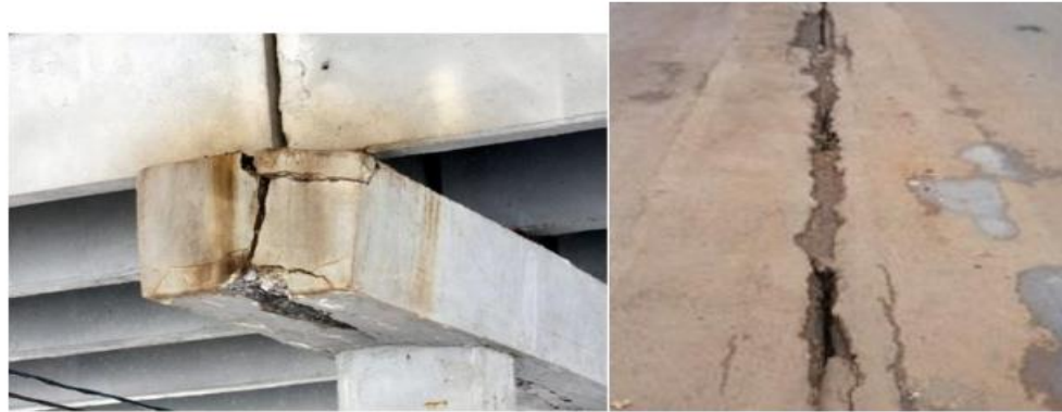
Figure 1: Fatigue crack on structural components [1].
